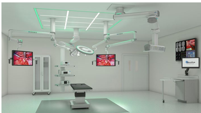
Figure 98 Example of a digital operating room (DOR) with 2 x ceiling mounted display screens, 1 x wall mounted display screen, 1 x standard surgical light, 1 x surgical light with integral camera, and 2 x medical services pendants (1 x with a vertical services head and 1 x with a horizontal services head)
