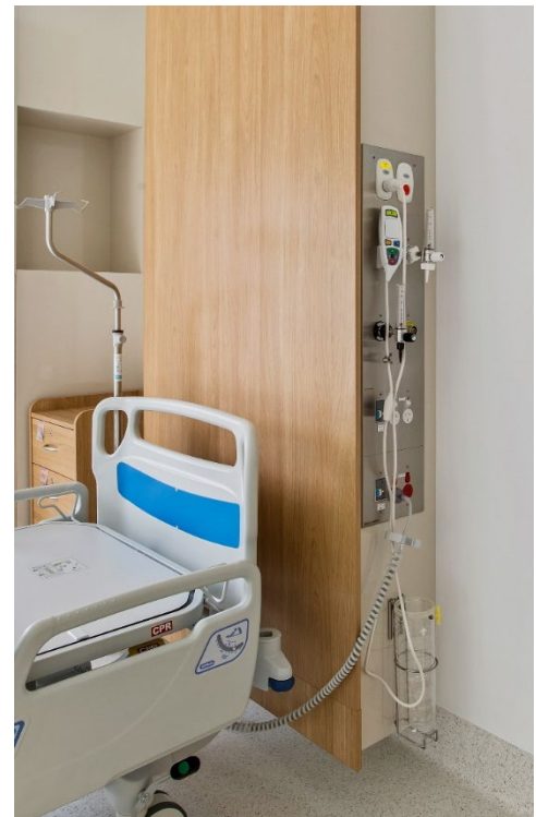
Figure 115 Example of a multi-row/vertical medical services panel arrangement on the outside of a bedhead joinery unit in a patient bedroom
