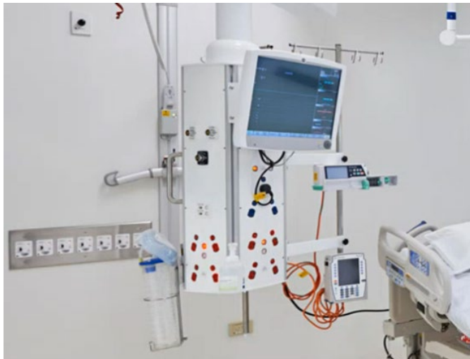
Figure 15 Example of services head accessories (equipment rails, IV poles, and brackets) and medical equipment (patient monitor and infusion pump) on a vertical services head in an Intensive Care Unit (ICU)
