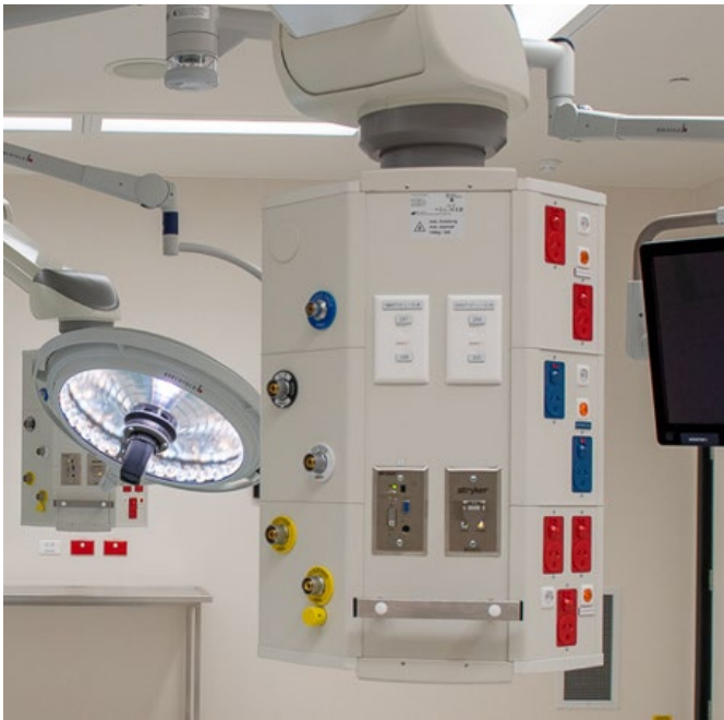
Figure 11 Example of services outlets (medical gas, power, communications, and audio-visual outlets) on a vertical services head, alongside surgical lights and a display screen in an operating room
