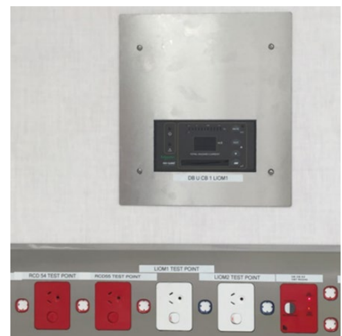
Figure 45 Example of a line isolation and overload monitor located above a medical services panel
