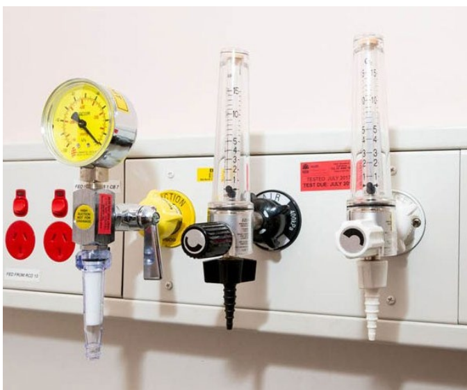
Figure 8 Example of services accessories (adapters and flowmeters) on a surface mounted medical services panel
