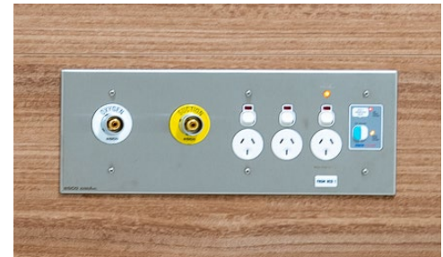
Figure 37 Example of a medical services panel with three white, non-essential power outlets
