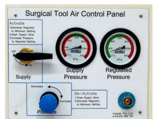
Figure 33 Example of a surgical tool air control panel on wall
