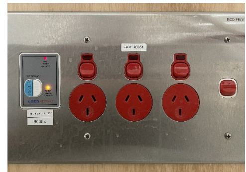
Figure 44 Example of an RCD to emergency power outlets on medical services panel
