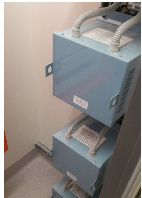
Figure 46 Example of an isolation transformer in an electrical cupboard
