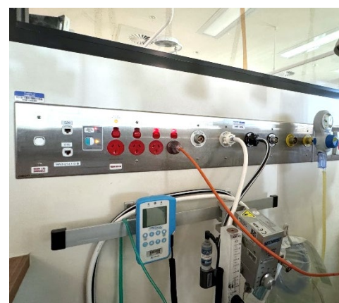
Figure 95 Example of a horizontal equipment rail in a neonatal care unit, mounted underneath a medical services panel, with medical air and oxygen mixer clamped on the rail under medical gas outlets
