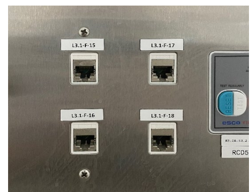
Figure 49 Example of a medical services panel with four RJ45 data outlets
