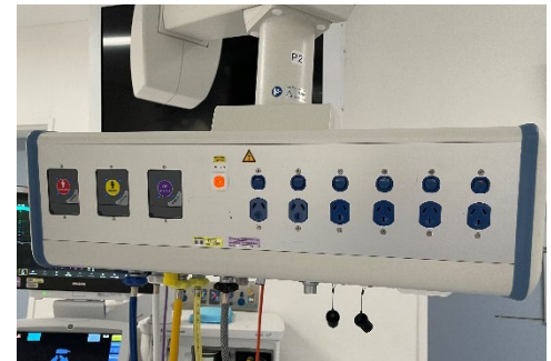
Figure 39 Example of a medical services pendant with six blue, UPS power outlets
