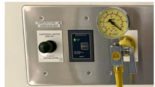
Figure 40 Example of a UPS status indicator on a medical services panel
