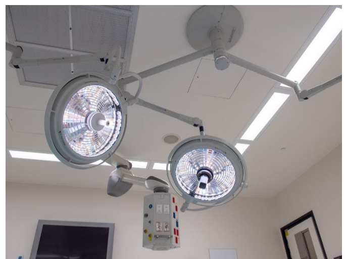
Figure 20 Example of DOR equipment (camera integral to operating light with connection to wall mounted display screen for live display)
