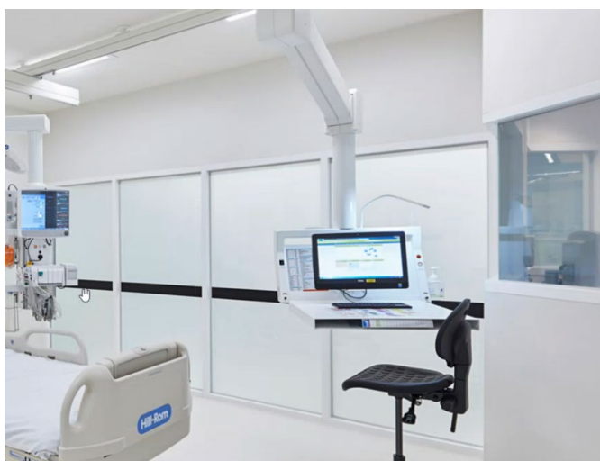
Figure 19 Example of workstation shelf with articulated task light and integral power and data connections, mounted directly to a connecting pole of a medical services pendant in an ICU bedroom
