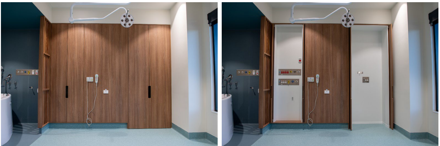
Figure 112 Example of concealed medical services panels in a birthing room in closed and opened position
