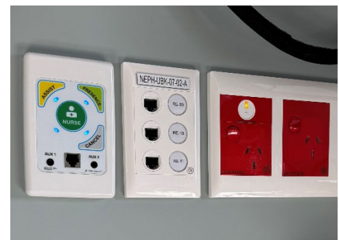
Figure 53 Example of a 6-gang surface mounted face plate on a medical services panel, with 3 x gangs used for data outlets and 3 x gangs used for associated labels
