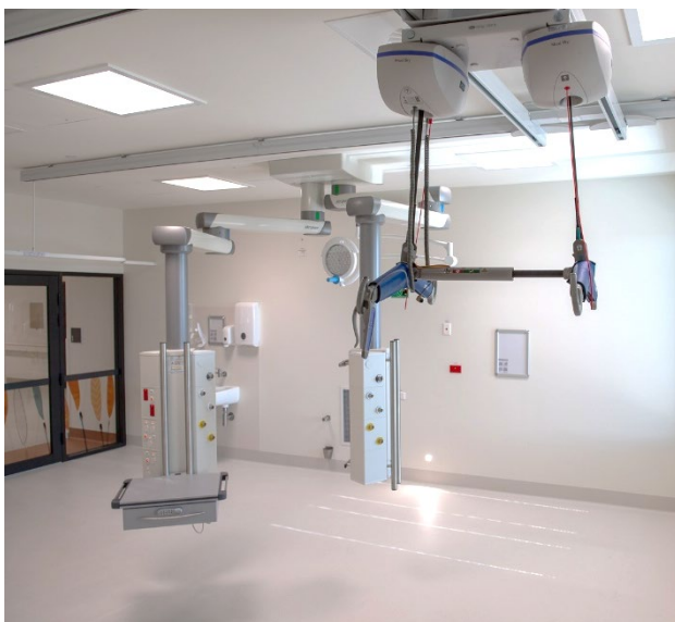
Figure 124 Example of double arm pendant in ICU bed room coordinated with a track for a patient lifter
