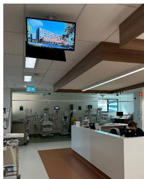
Figure 83 Example of ceiling mounted nurse call annunciator display screens in front of a staff station
