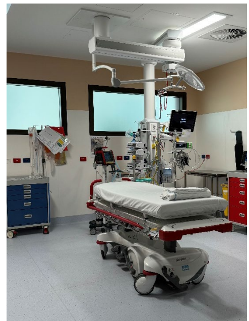
Figure 126 Example of a single arm medical services pendant at the head of the bed in a resuscitation bay. The pendant has been coordinated with a ceiling mounted procedure light that is mounted behind it
