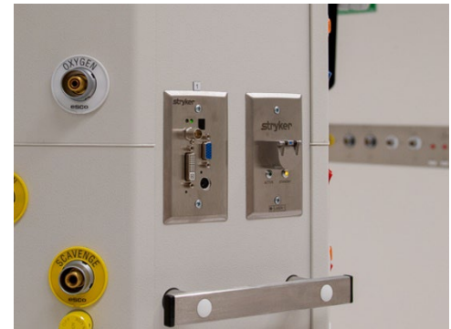
Figure 50 Example of audio-visual outlets (including VGA and DVI outlets) on a medical services pendant
