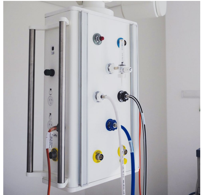
Figure 12 Example of services outlets (power, data and medical gas outlets), services accessories (flowmeter) and service head accessories (equipment rails) on a vertical services head
