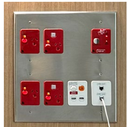
Figure 38 Example of a medical services panel with four red, emergency power outlets
