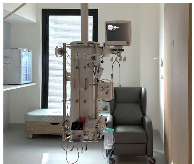
Figure 14 Example of services head accessories (equipment rails and brackets), medical equipment (patient monitor, medical air/oxygen blender, and neonatal ventilator), and on a vertical services head in a Neonatal Intensive Care Unit
