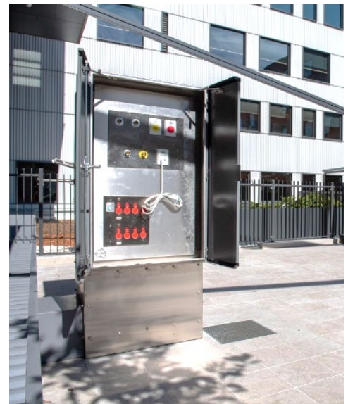
Figure 118 Example of an outdoor medical services panel in a courtyard associated with an intensive care unit
